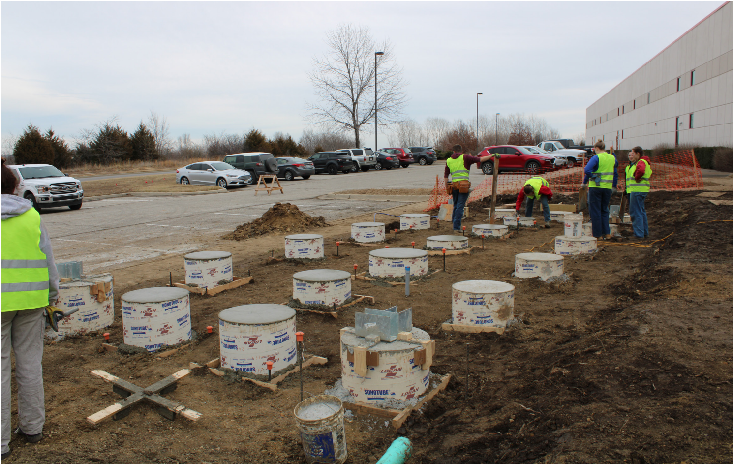
Haven Studio, photo of the piers and pier connectors that hold the floor structure off the ground..
