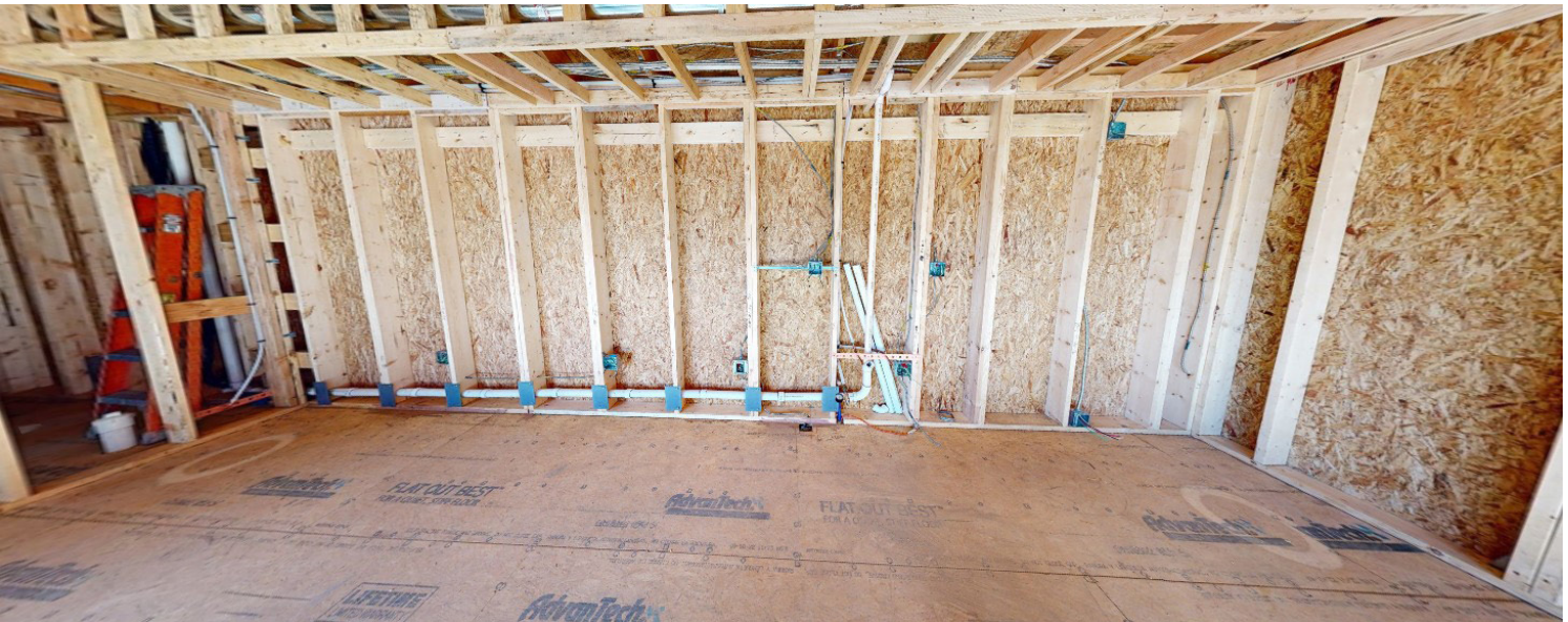
Haven Studio, view of the interior wall framing showing the doubled studs.
