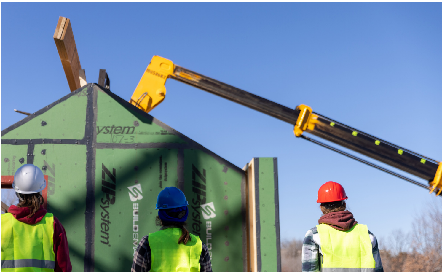
Haven Studio, photo of installing the ridge beam onto the Build SMART prefabricated wall panels.
